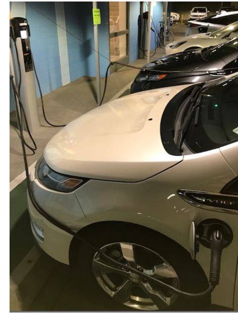
EV Parking in SMC underground garage
